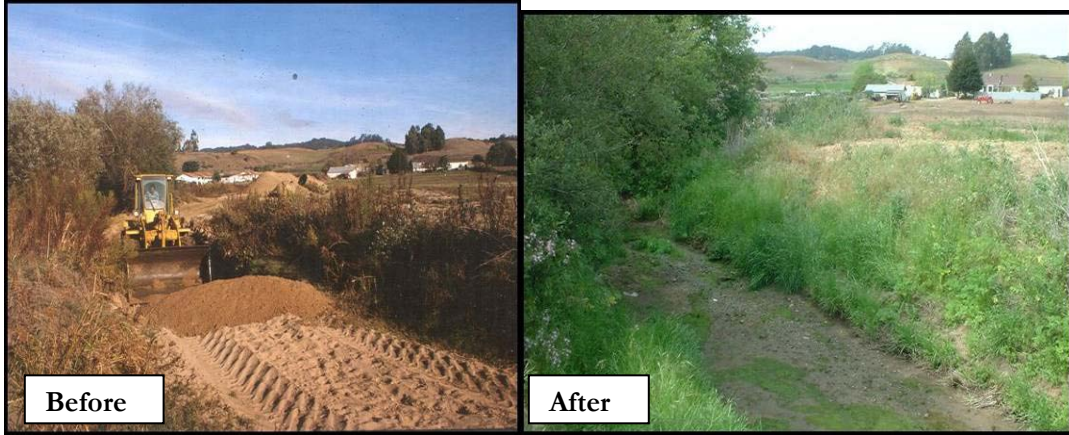
Example above: One-time removal of sediment causing damage to banks
