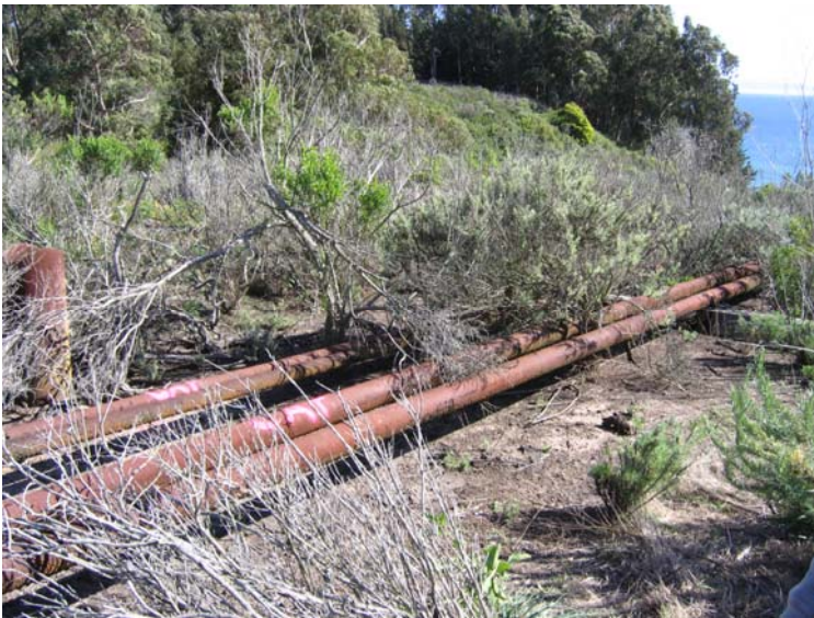
Pipeline on Eagle Canyon Ranch
